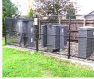
How substations should be - safe and secure
